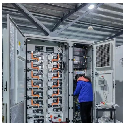
OASIS 60 Battery Cabinet: Scalable Energy Storage for Businesses
