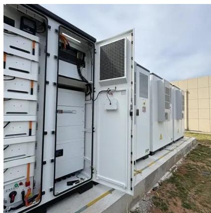
Huijue lithium iron phosphate outdoor power cabinet
