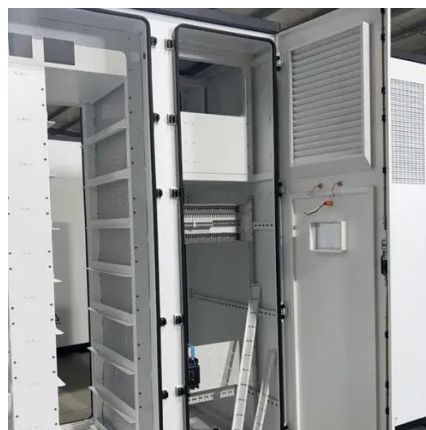
Male Modular Outdoor Cabinet 350kw , MSC Industrial Supply Co.
