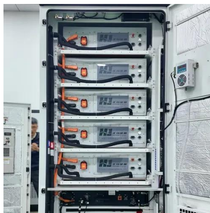
Growatt 5kW Inverter , Stackable , Off-Grid , 48V
